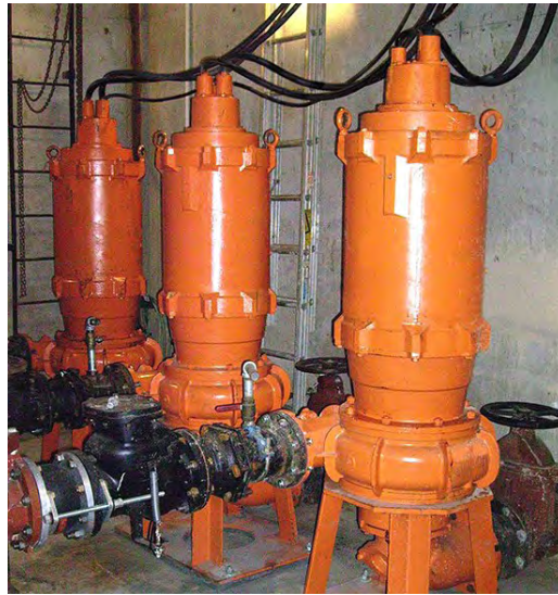
Figure 3-12 Dry Pit Submersible Pumps (Chicago Pump)
