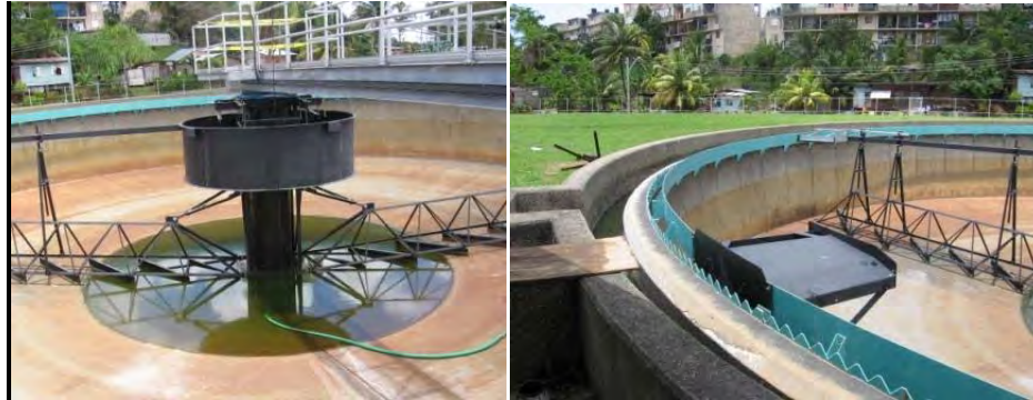
Figure 3-16 Recently Refurbished Primary Clarifiers at San Fernando WWTP
