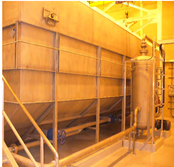
Figure 3-21 Stainless Steel DAF Tank
