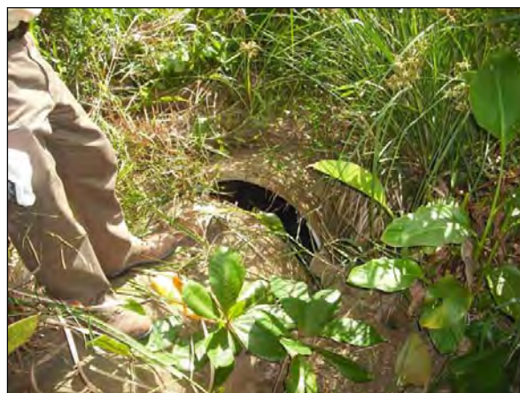
Figure 3-5 Section of Trunk Sewer along Vistabella River Showing Open Joint
