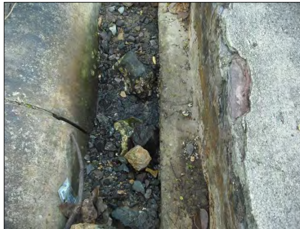
Figure 3-4 Section of Trunk Sewer Along the Sea Wall Showing Possible Points of Inflow at Pipe Joints
