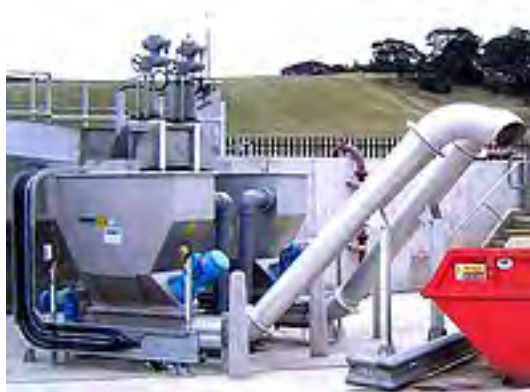
Figure 3-15 Screenings Compactor (Courtesy of Huber Technology)
