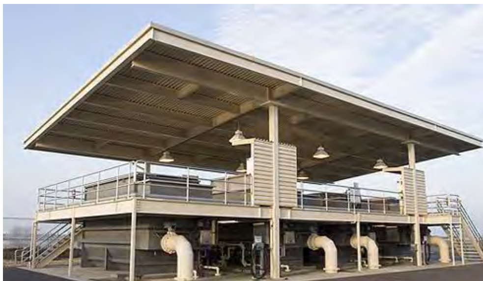
Figure 3-19 Cloth Media Filtration Plant (Courtesy of Aqua-Aerobic Systems)
